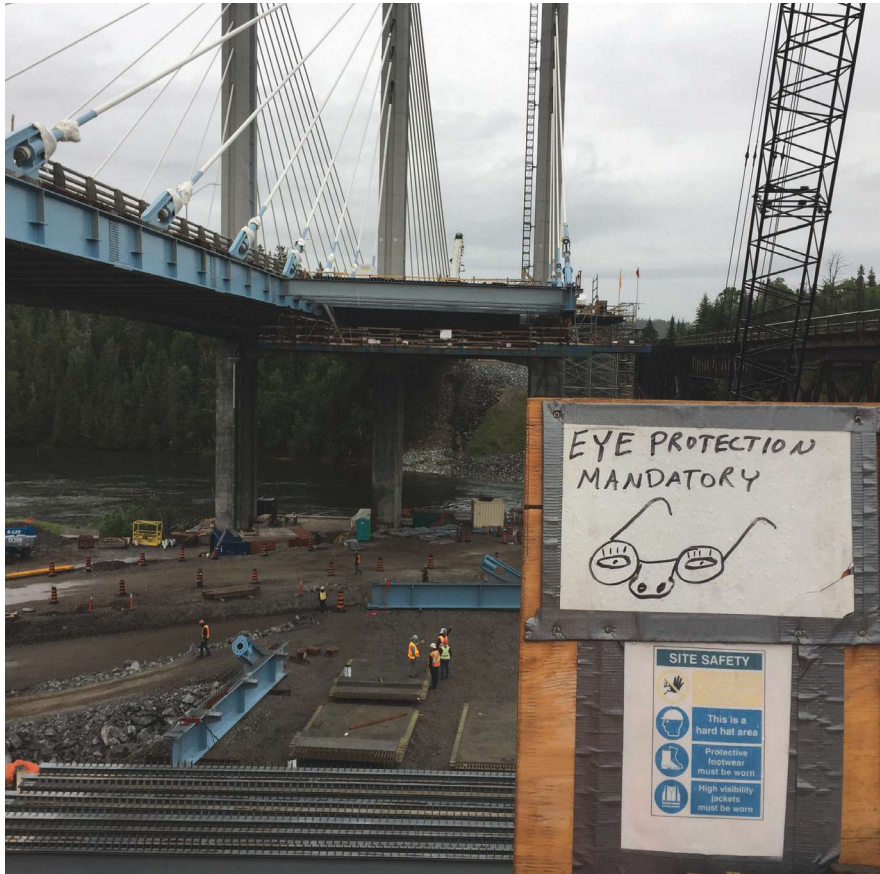
Fig. 1: Sign showing required safety controls at the Nipigon River Bridge Project in Ontario, Canada
